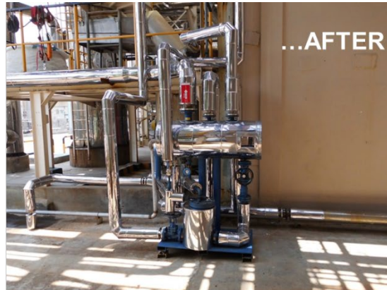
Mechanical Pump with compact condensate receiver tank Removed bigger condensate tank, less space
