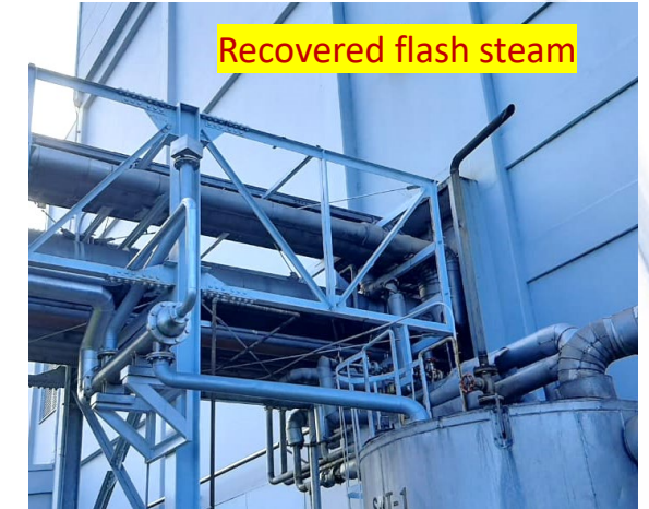
Flash Steam Condenser
