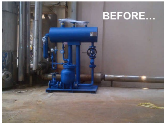
Sentrifugal pump and bigger condensate tank
