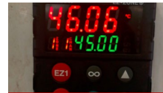
Hot water temp.
