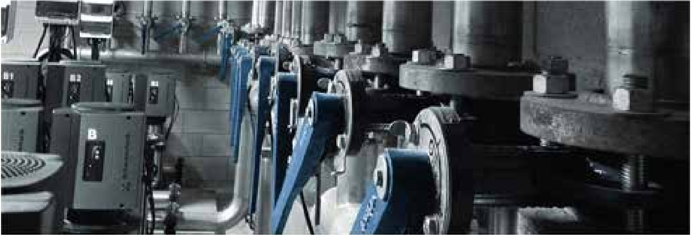
Water supply plant room in a commercial building.
