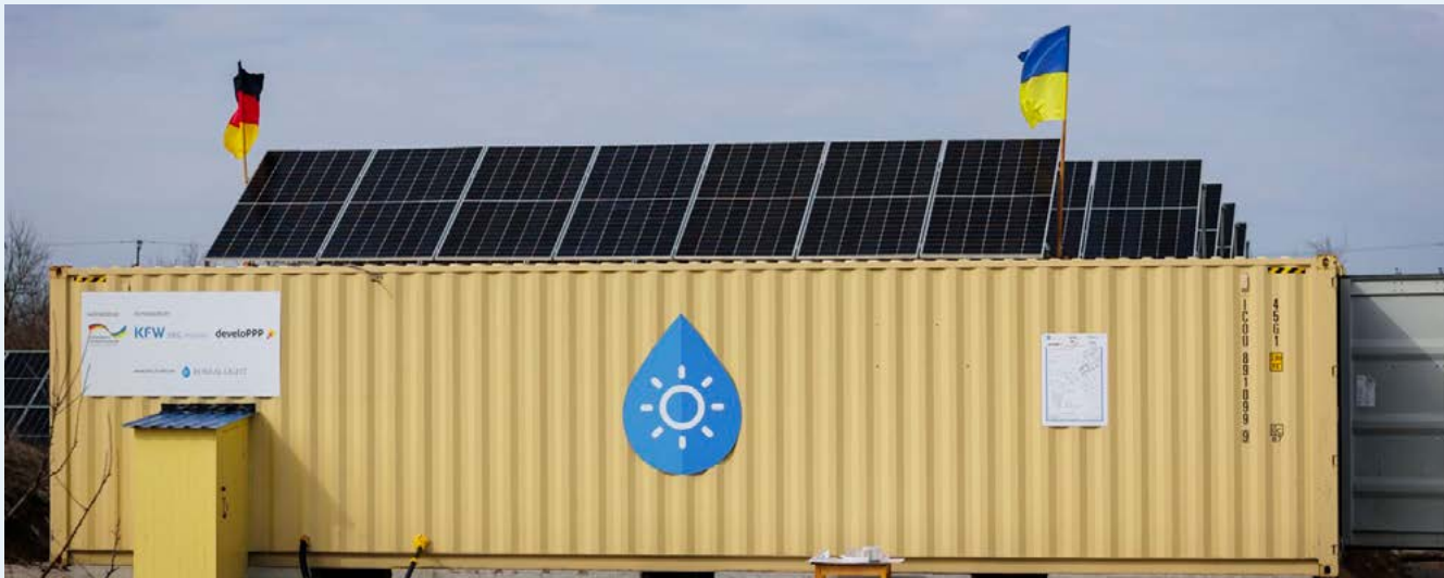
The desalination system is partly solar-powered, meaning that it's powered by the sun 10-12 hours during a typical summer's day, and 4-6 hours per day during the winter.
