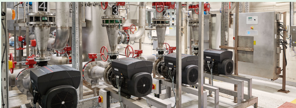
The Grundfos beverage network supply pumps.
