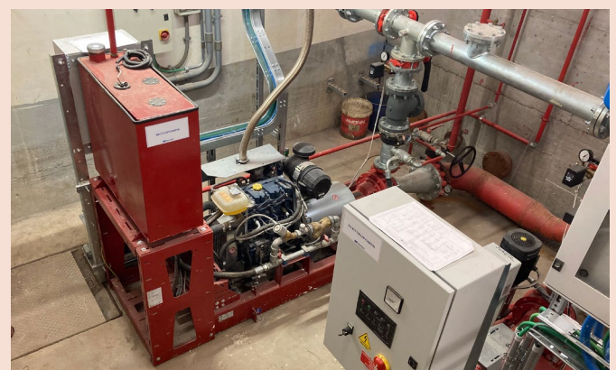
Firefighting unit consists of an electric pump and motor pump
