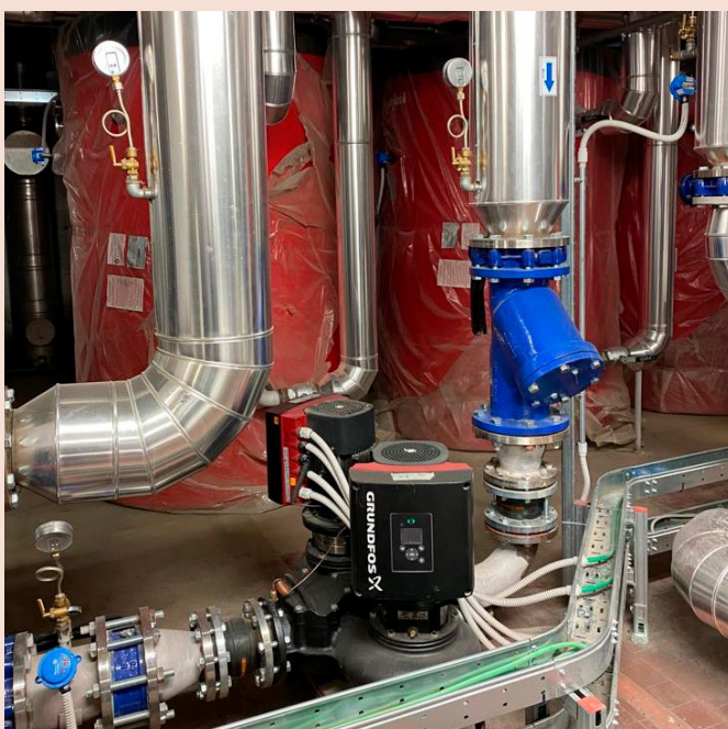
Circuit with domestic hot water heat exchanger was made using TPE pumps
