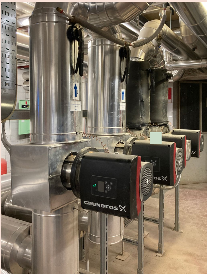
Secondary circuit water cooler and refrigeration unit was made using TPE pumps
