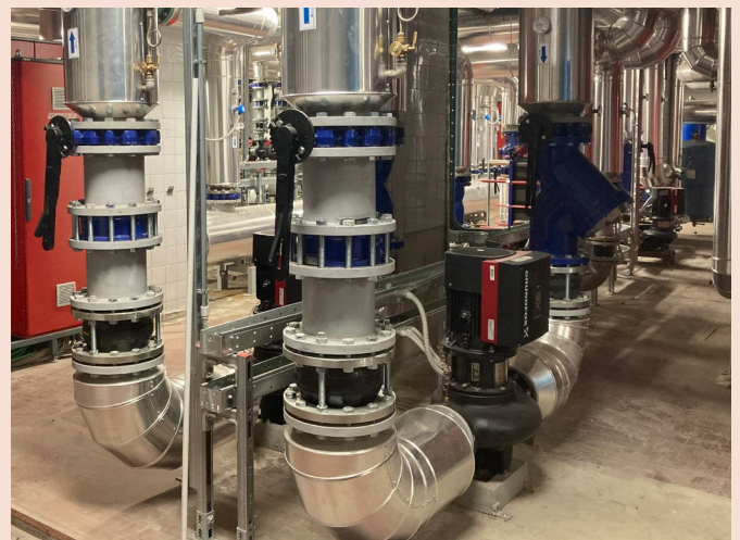
Primary heat pump circuit consisting of TPE pumps
