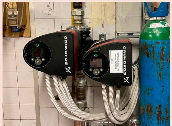
The twin domestic hot water recirculation pump is a Magna3 model
