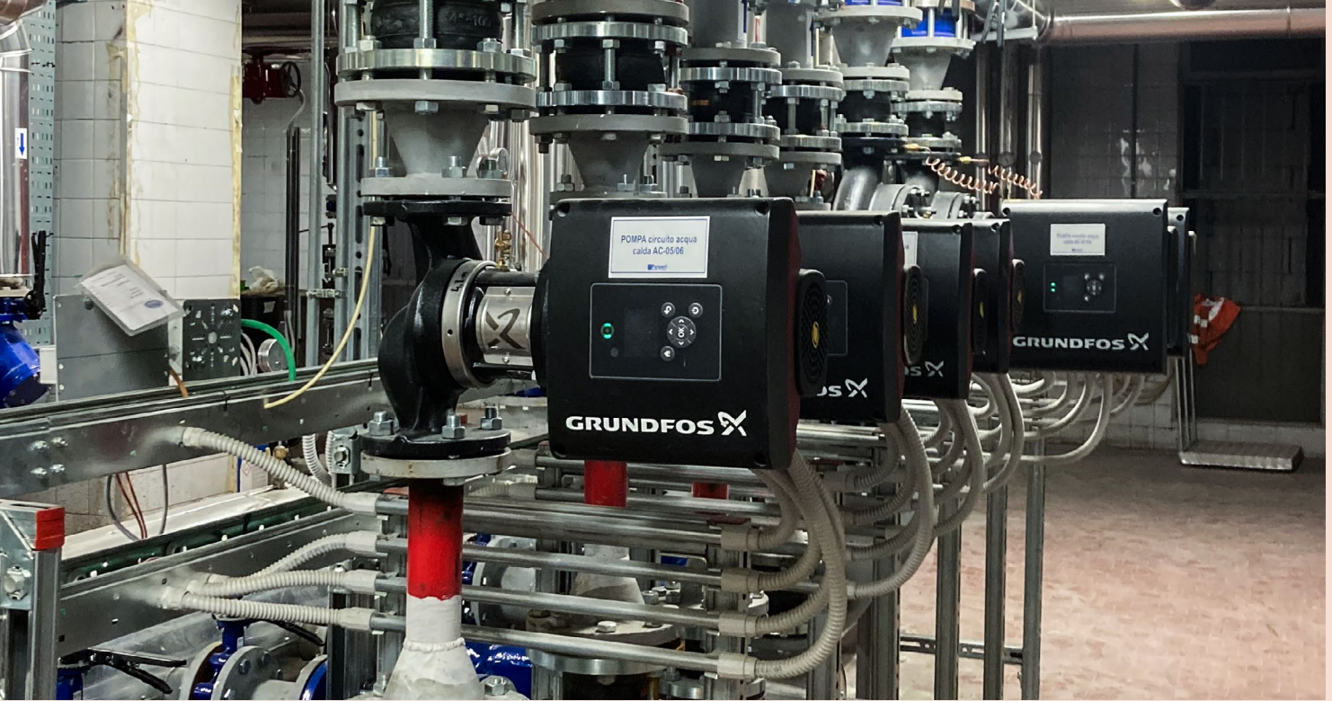
Secondary heating circuit consisting of TPE pumps
