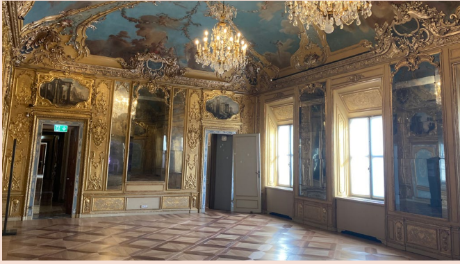
In one of the building's principal rooms we focused on working on the floors: installation of the air conditioning was completed with a number of fan coils under the window
