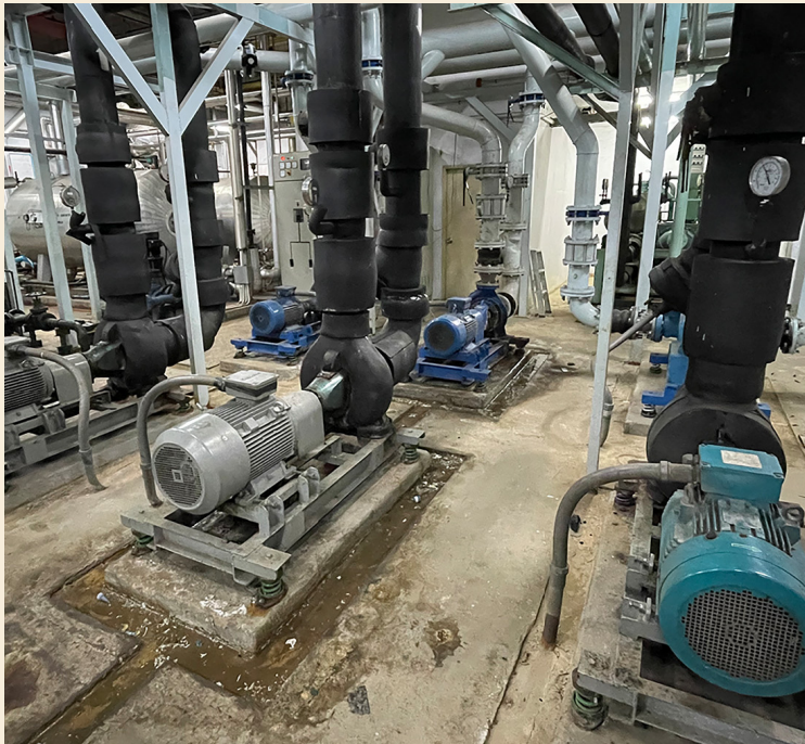
Old installation of chiller pumps
