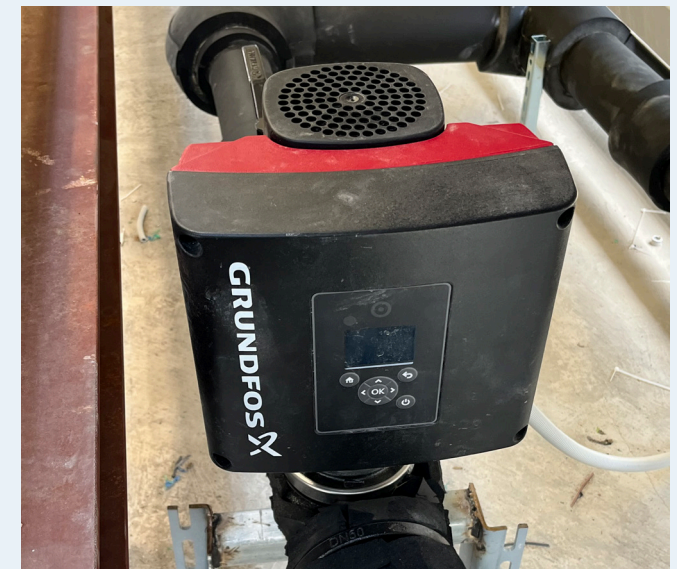
A TPE3 circulator powers the primary circuit.
