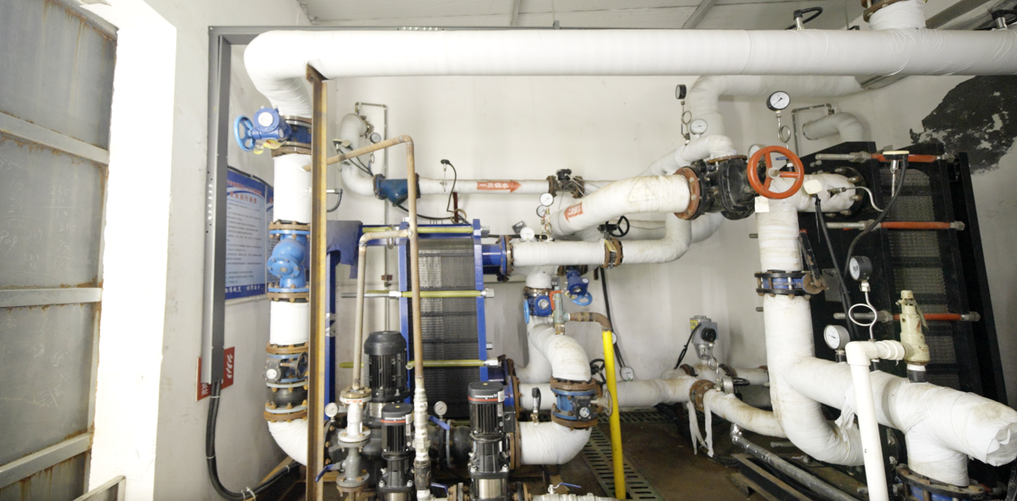
Source pump and de-coupler in the sub-station
