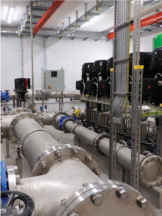
The connections to the two pressure boosting systems and the diaphragm expansion tanks are located in the basement of the underground reservoir
