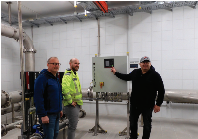
Monitoring the pump technology – from left to right: Bernhard Sedlmeier, Water Engineer at Stadtwerke Schongau; Dipl.-Ing. (TUM) Florian Hiemer, Technical Plant Manager at Stadtwerke Schongau; Maik Wötzel, Senior Sales Engineer at Grundfos GmbH
