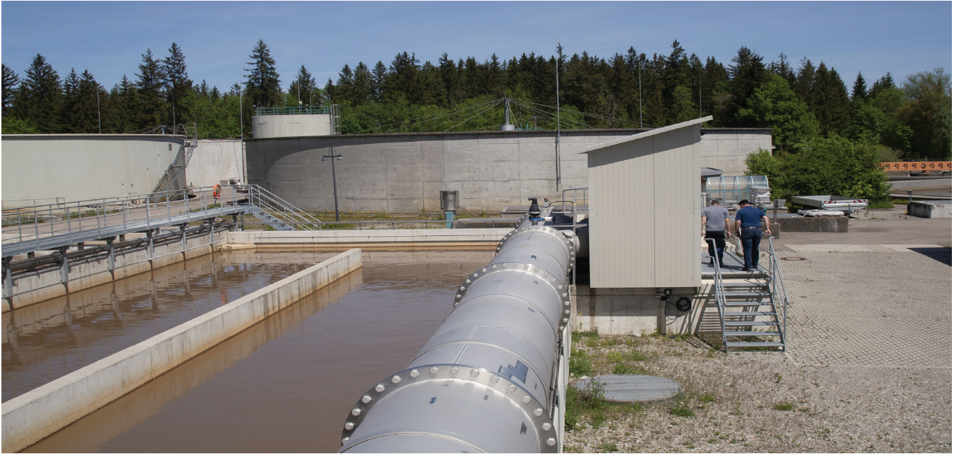
Denitrification with recirculation and discharge from process water treatment. Tank size: 3,750 m 3
