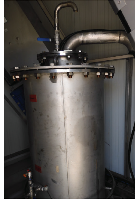
Two propeller pumps are installed in the fixed anchorage points/fittings.
