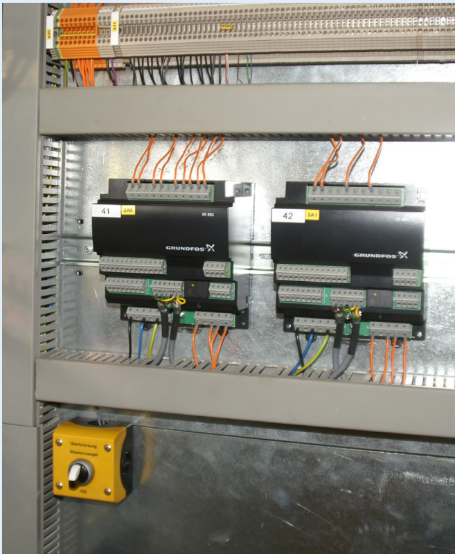
New CU 352 control unit - The pressure boosting system has been running without any failures since July 2022.
