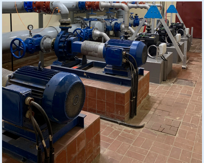
Booster in the rebuilding phase – old pump technology in front, 3 new NBE 65-200/198 at the rear (June 2022)
