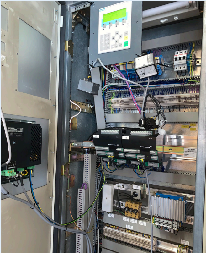
Old control technology in the control cabinet during the conversion phase
