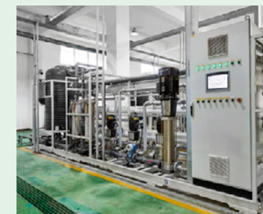
Just a few of many Grundfos pumps (these are CRN and CMs) in the WELLE membrane treatment facility.
