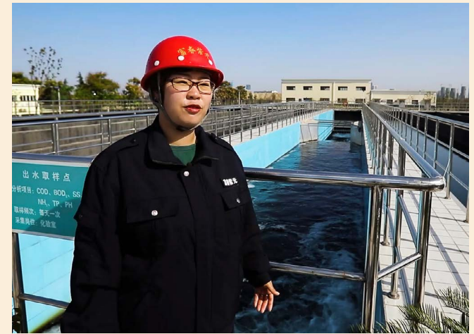
"As the biggest wastewater plant in Xiangyang, our key concern is to make sure the operation is safe and efficient, including in the treatment and emission process,"
