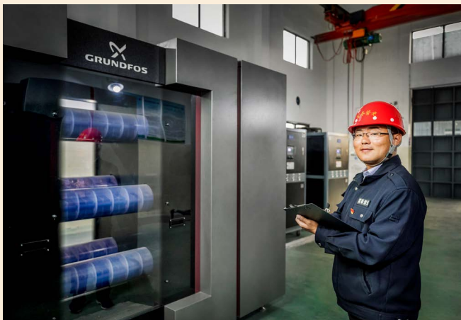
"It's proven that we've made the right call to choose Grundfos Selcoperm," Xu Feng , project manager at the wastewater plant.
