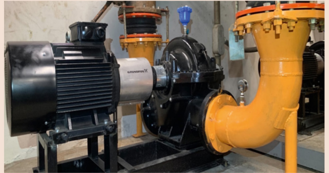
Grundfos Chiller Condenser Water Pump
