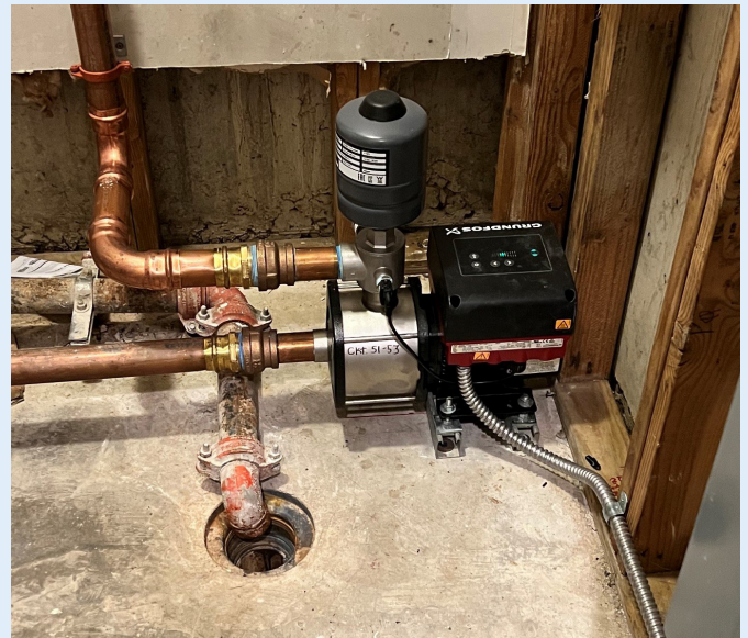
Grundfos CMBE 10-54 pumps for the Retreat at Tiffany Woods.
