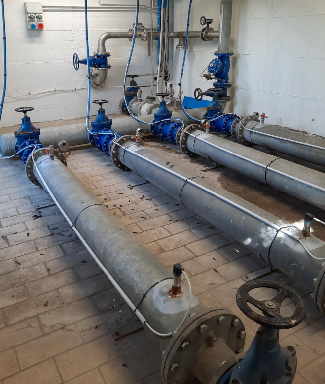
Booster station with motor replacement.
