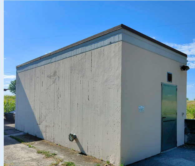
Exterior of the electric panel room at the Torbole Casaglia (BS) waterworks booster station.
