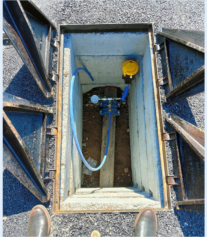
Inspection shaft: Critical Point pressure sensor.
